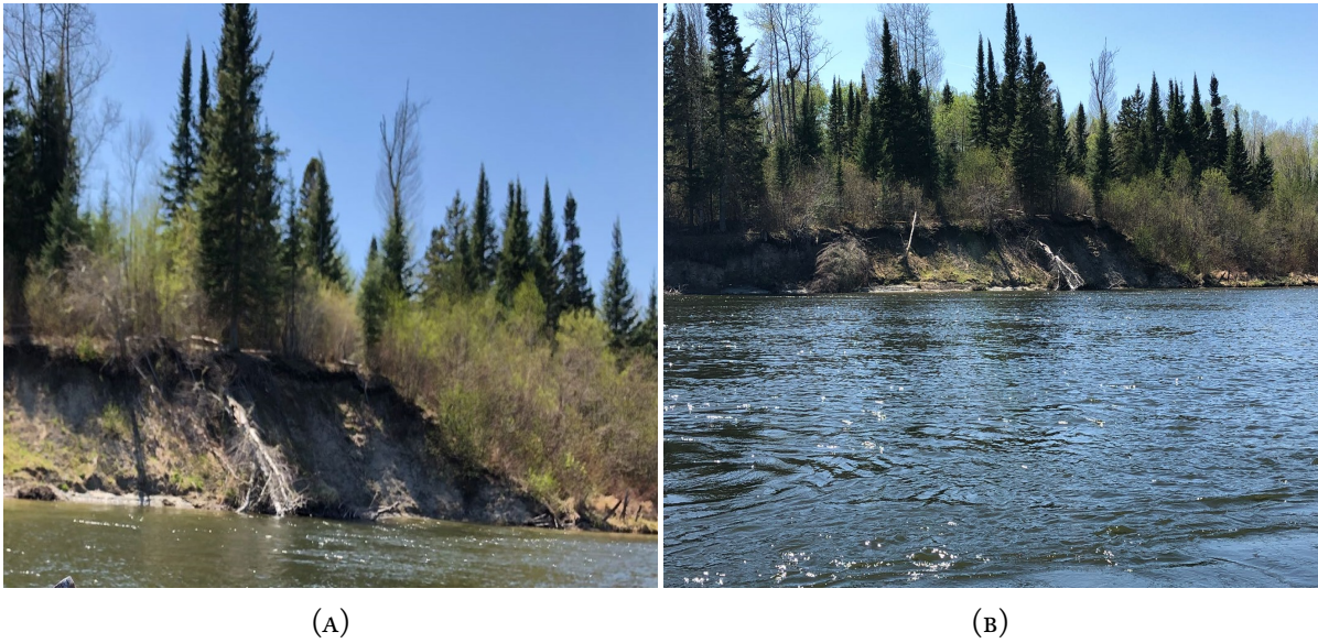
FIGURE 3.8: Evidences of slope instabilities on the Nipigon river banks
