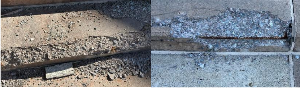
Figure 2.5: Damage to stairs at Lakehead University caused by freezing and thawing
