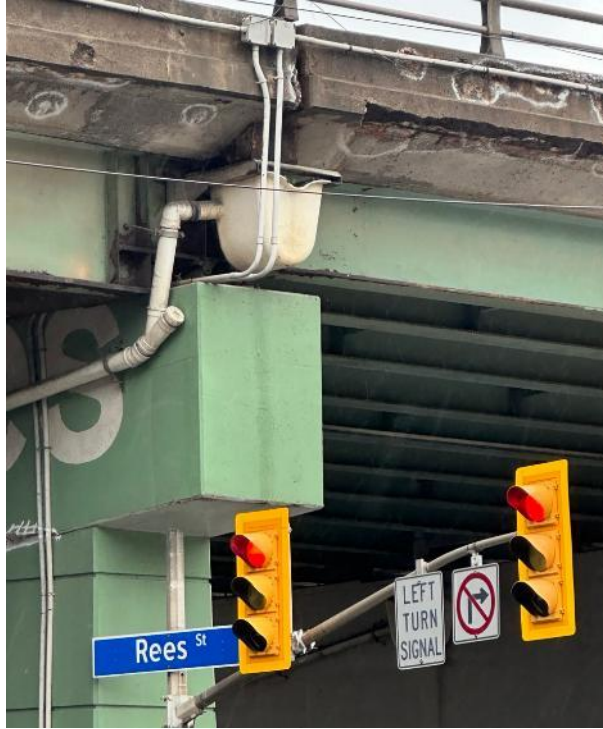
Figure 2.4: Chloride attack on reinforced concrete (Rees st, Toronto)
