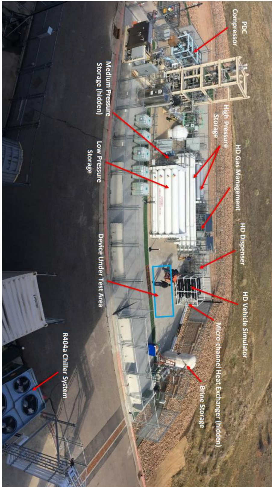
Fig. 19. NREL HD Fast Flowing Test Facility [37].
