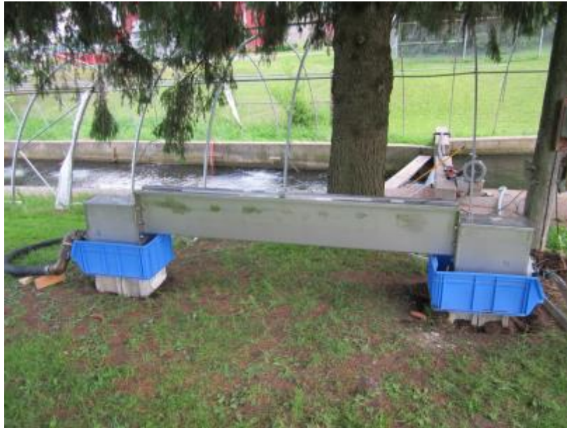
Figure 8: Photograph of the installed UV lamp at Lyndon Hatchery.
