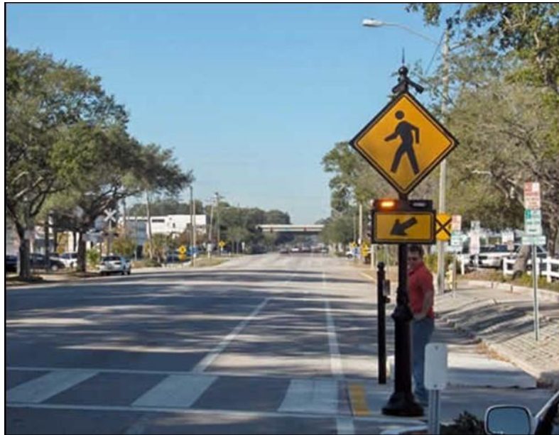
Figure 6.21: Example of a RRFB being activated by a pedestrian (FHWA, 2017b).
