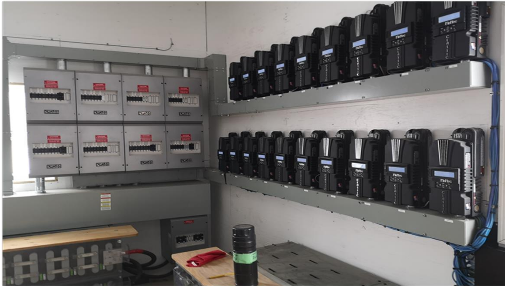
Figure 4. LDMLFN PV-BESS system interior (Lac des Mille Lacs First Nation).
