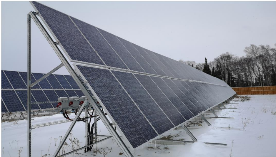
Figure 3. LDMLFN PV-BESS system exterior (Lac des Mille Lacs First Nation).
