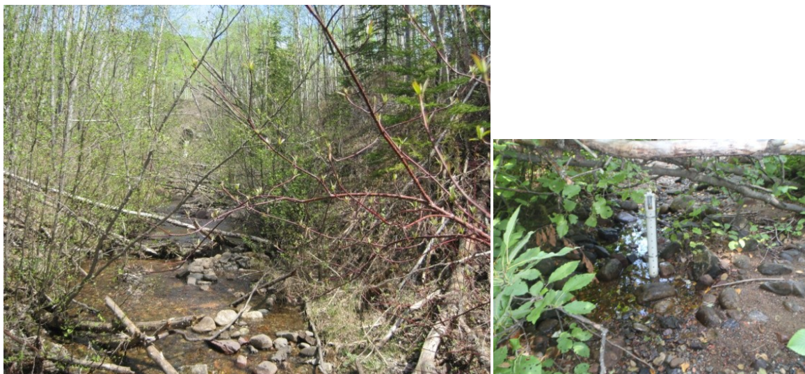
Figure 3.2. Photo of reach 1, (left) the old straightened channel, and location of site 1, (right) within reach 1 near the culvert below the railway.
