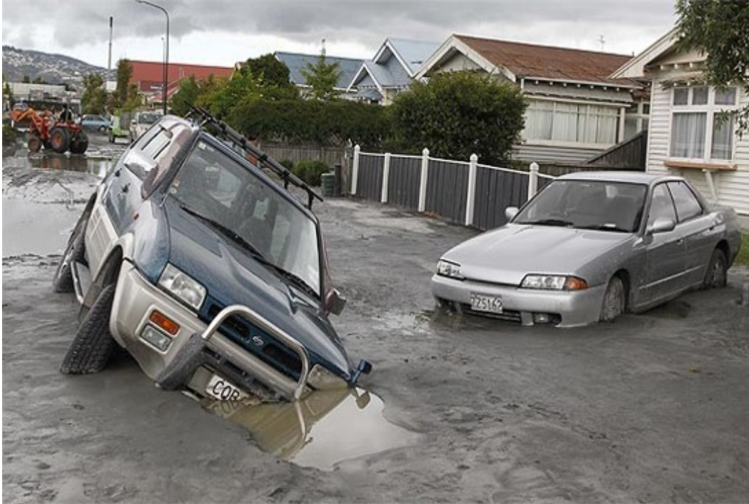
Figure 1.3: Road damaged due to soil liquefaction at Christchurch, New Zealand (2011) (National Academies of Sciences et al., 2016)
