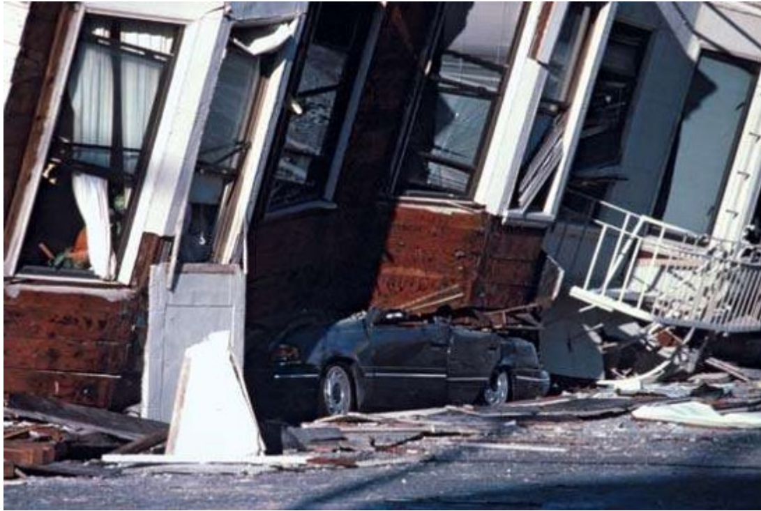
Figure 1.2: Building collapse at California due to soil liquefaction in 1989 (National Academies of Sciences et al., 2016)
