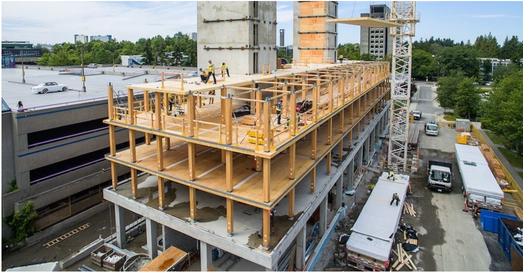
Figure 3: 2016 construction of UBC Brock Commons' tall wood residence(UBC Public Affairs) by KK Law. (Source from: https://dailyhive.com/vancouver/bc-building-code-tall-wood-buildings-2019 .)
