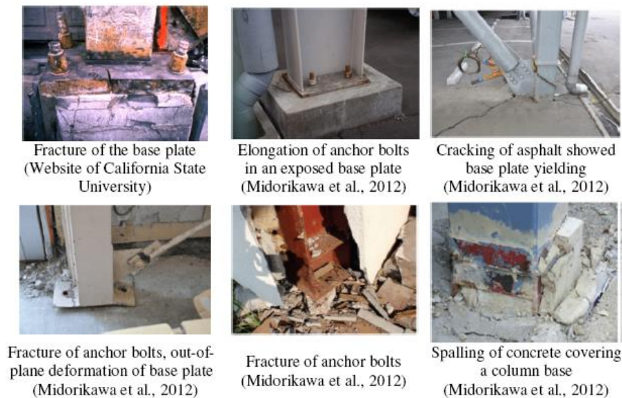
Figure 2.3 Base connection failure observed in past earthquakes
