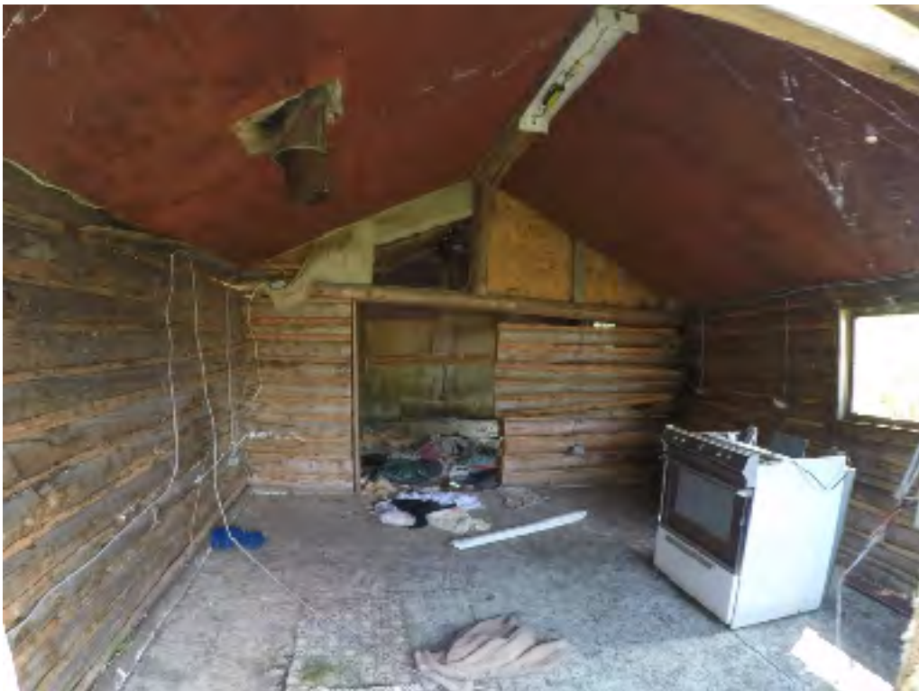
Figure 6.30, View from inside cabin in Area III, note vinyl flooring, electric oven, chainsawed-addition, fluorescent lighting and flue for wood-stove.
