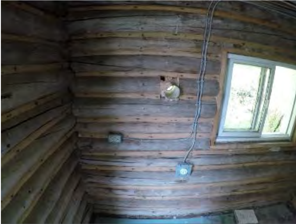
Figure 6.31, View from inside cabin in Area III, electric wiring laid overtop walls, sliding screen window present in cabin.
