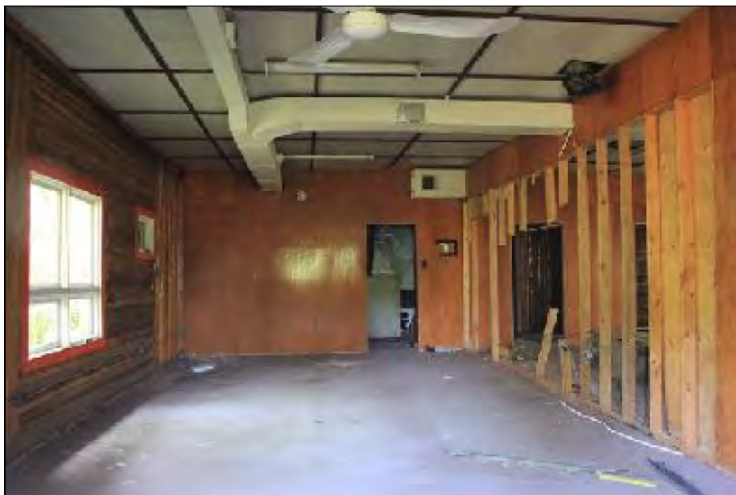
Figure 6.39, Interior of The New School, modern attributes; H-vac ducting, florescent lighting, ceiling tiles, partitioned rooms, sliding windows, carpeted floor, and electric ceiling fan.
