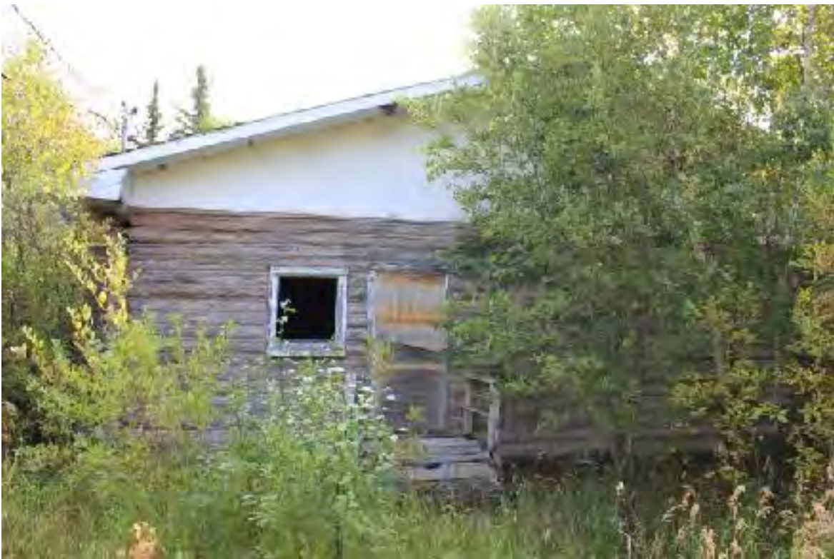
Figure 6.37, The New School as viewed from exterior, east facing wall. Large amount of foliage and regrowth surround the structure.
