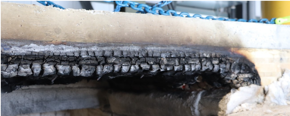
Figure 4.45: Horizontal charring behaviour at the supports.
