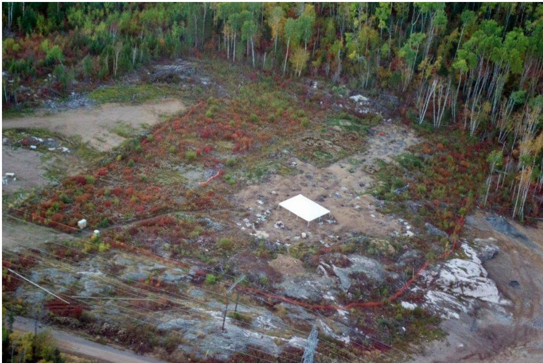
16) Top: View of bridge construction, looking east from the Mackenzie I site. Reprinted with permission by Markham (pers. comm., 2015). Bottom: Aerial view of the Mackenzie I site. Reprinted with permission by Norris (pers. comm., 2015).
