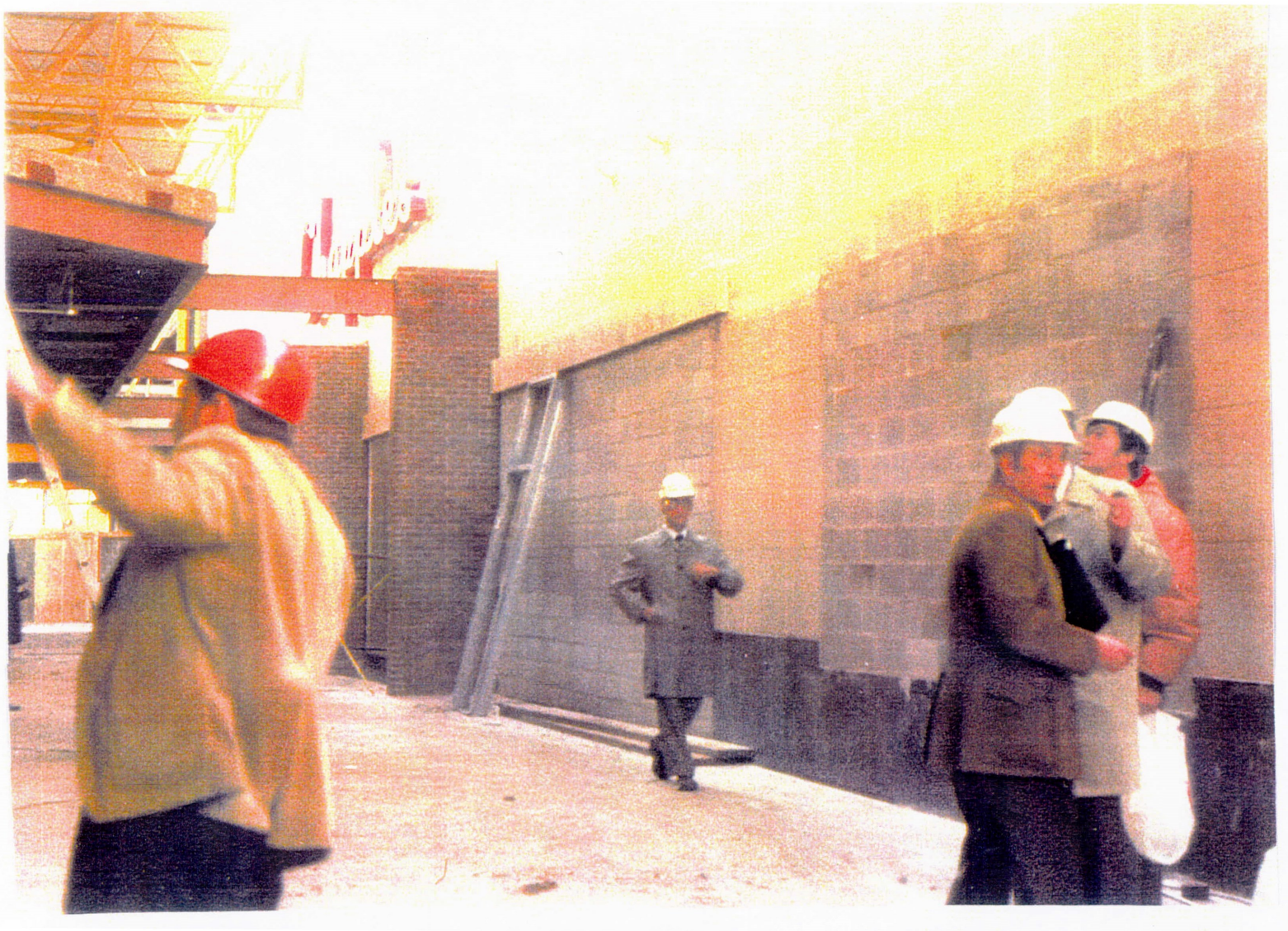
Bones McCormack (in the centre of the picture), inspects the construction of the Fort William ward revitalization project, circa 1979. (Photo: Murray Hamilton).
